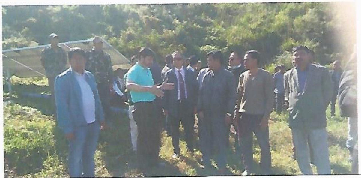
Solar water Pump Installed under NEC project "Model Horticulture Centre at Ngarumphung, Ukhrul District, Manipur"
