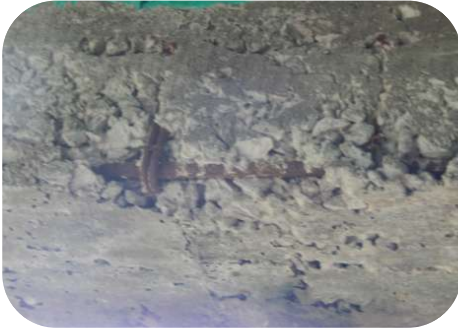
View of reinforcement expose in beam
