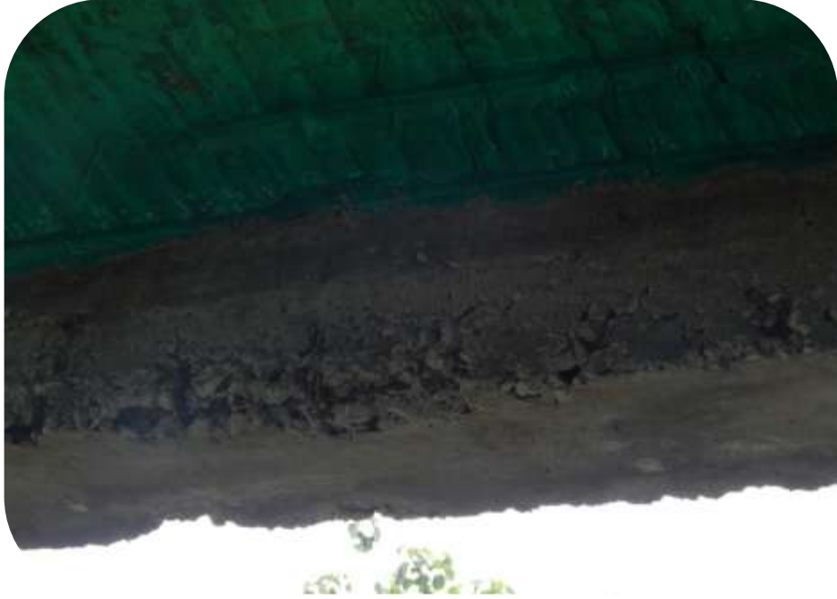
View of reinforcement expose
