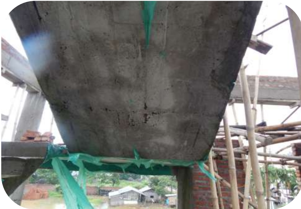
View of reinforcement expose in staircase
