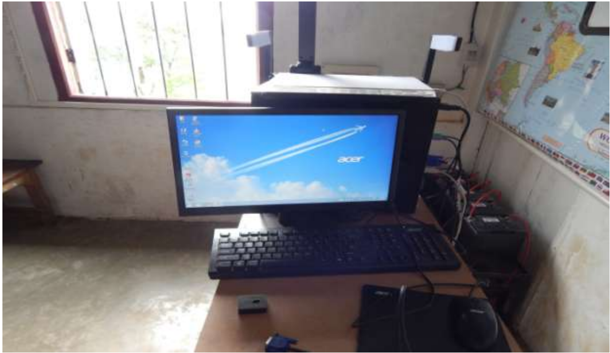
View of UPS,Desktop PC at Government Higher Secondary School at Serchip ,Mizoram
