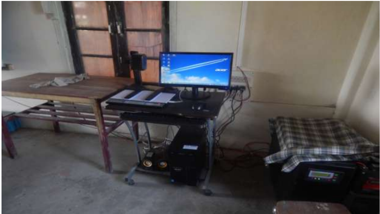
View of UPS,Desktop PC,Visual presenter at Government Higher Secondary School at Lunglei District,Mizoram.
