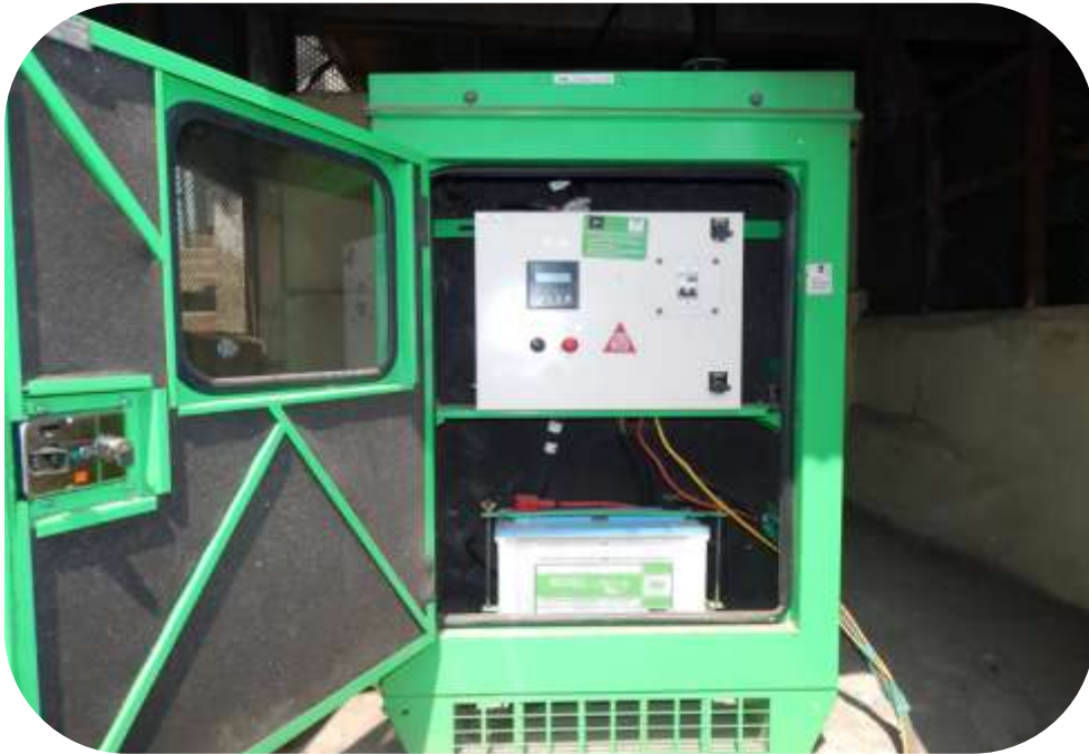
View of DG Set
