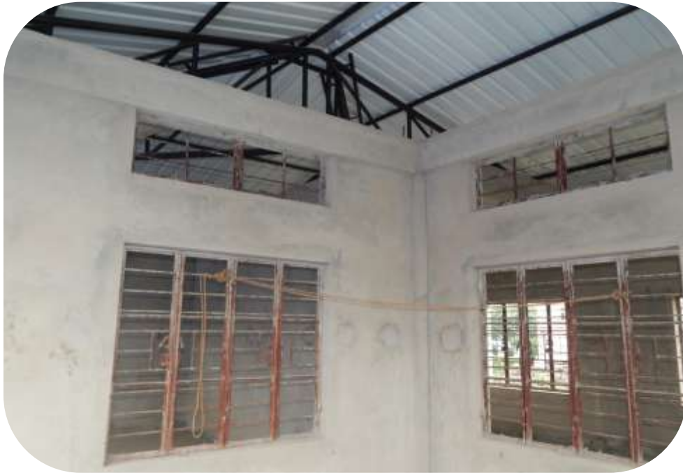
View of Window, truss and room in first floor of 50m range
