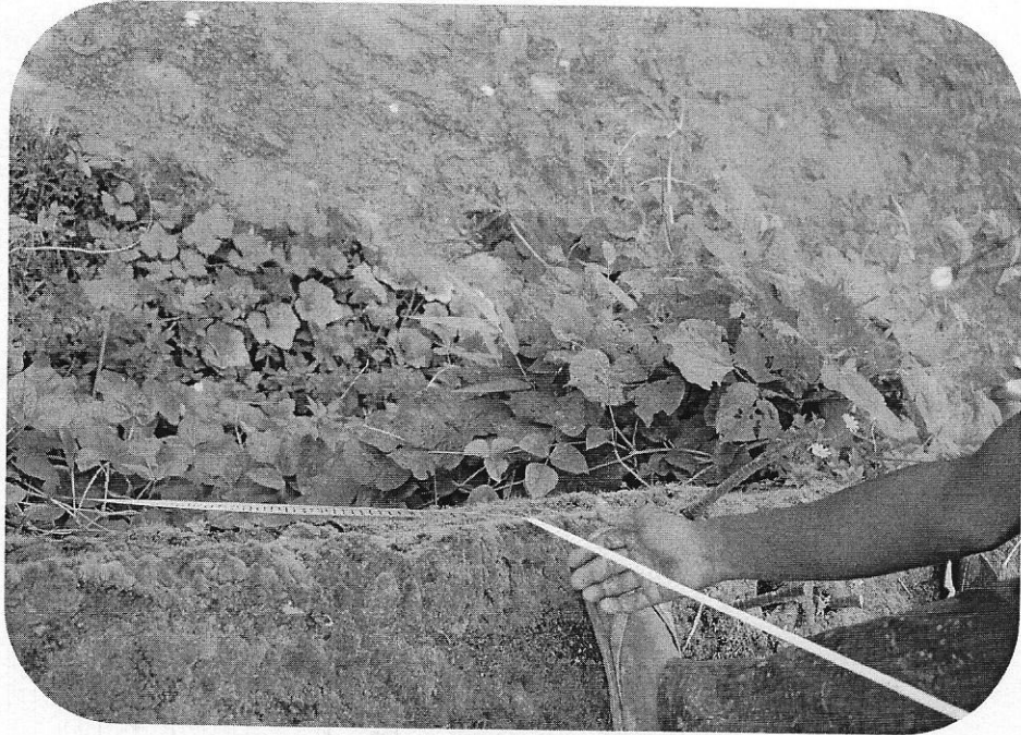
view of Consultant measuring the height of the Retaining wall at the original site
