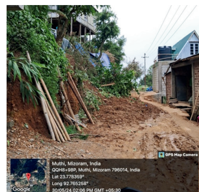
Fig. 2- Landslide in the eastern site of the locality. Muthi, May. 2024
