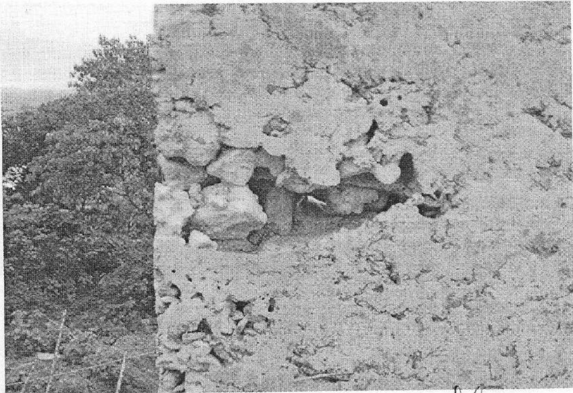
Photo showing the quality of casting in a column. Reinforcement exposes.
