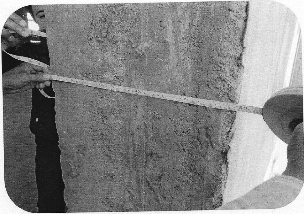
view of column size.
