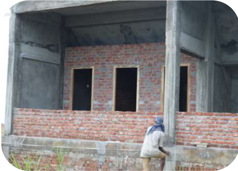
View of Toilet inside the Bay and below view of size of the column
