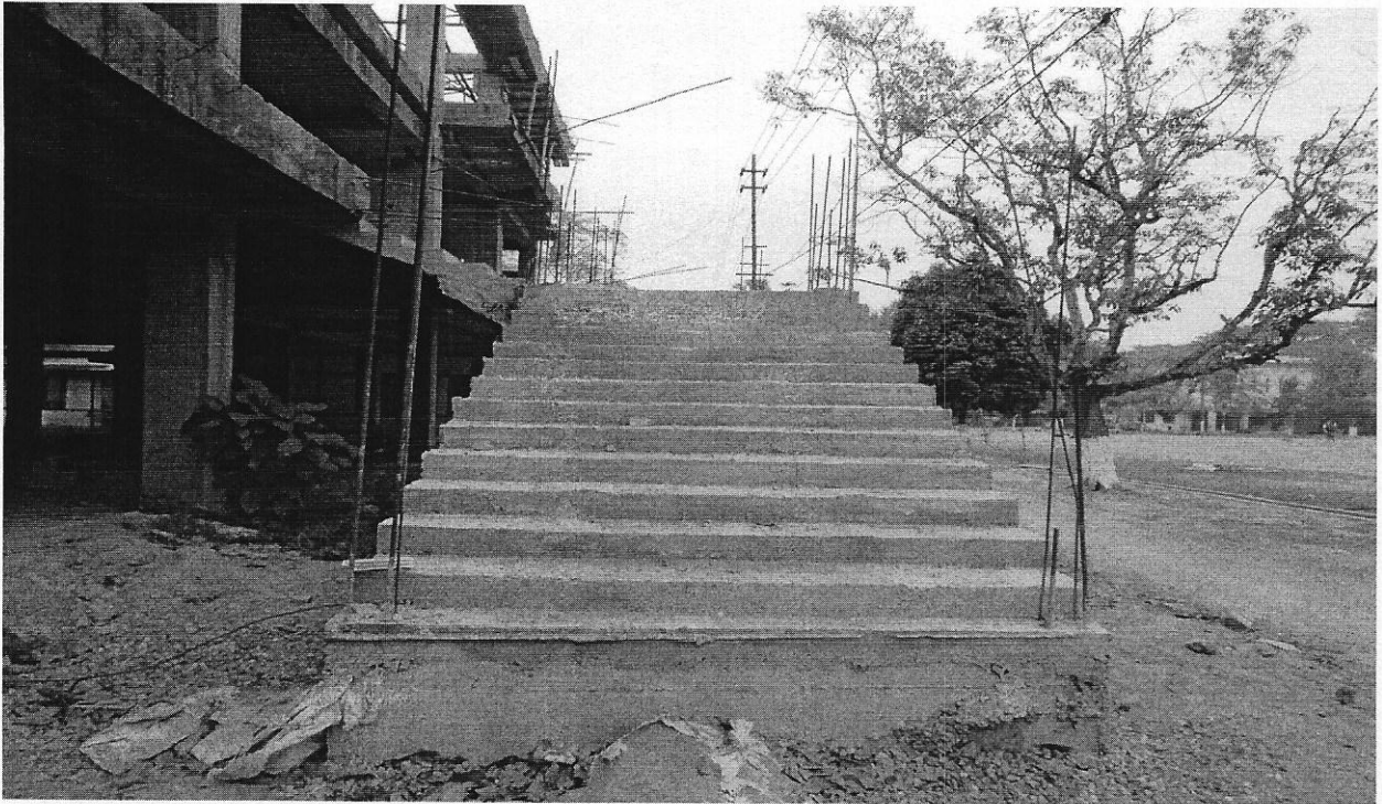
View of Staircase in front of the.C.C.(G+2) building for Seminar Hall, Computer Centre and facilities for Car parking at Darrang College,Tezpur,Assam
