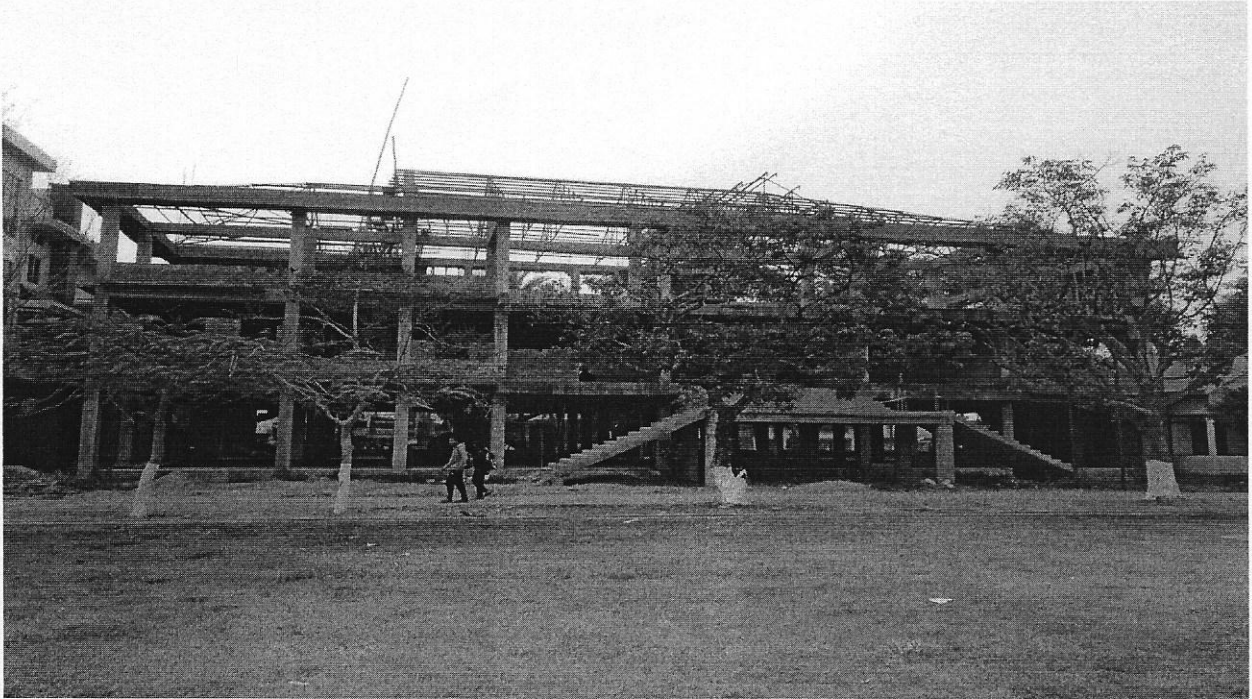
View of Construction of R.C.C.(G+2) building for Seminar Hall, Computer Centre and facilities for Car parking at Darrang College, Tezpur, Assam
