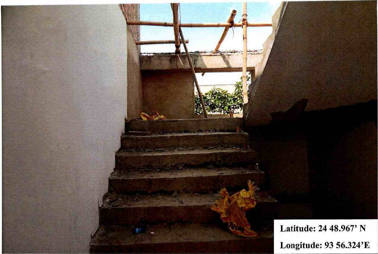
View of the staircase towards the 2 nd floor level of the building “Construction of Boys hostel (RCC+G2) with Toilets at Jawaharlal Nehru”, Manipur.
