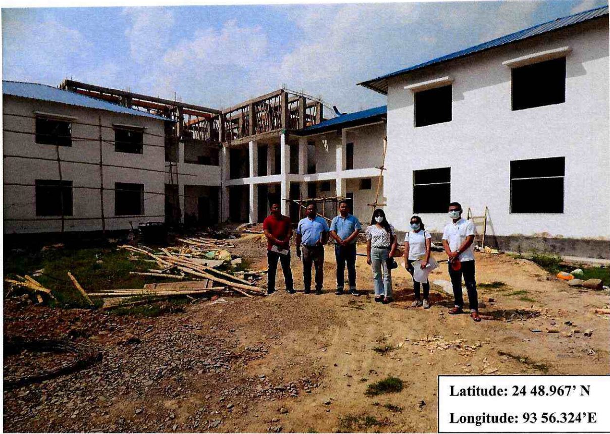
Photo of the inspection team along with official of the Implementing department at the project site for the “Construction of Boys hostel (RCC+G2) with Toilets at Jawaharlal Nehru”, Manipur.
