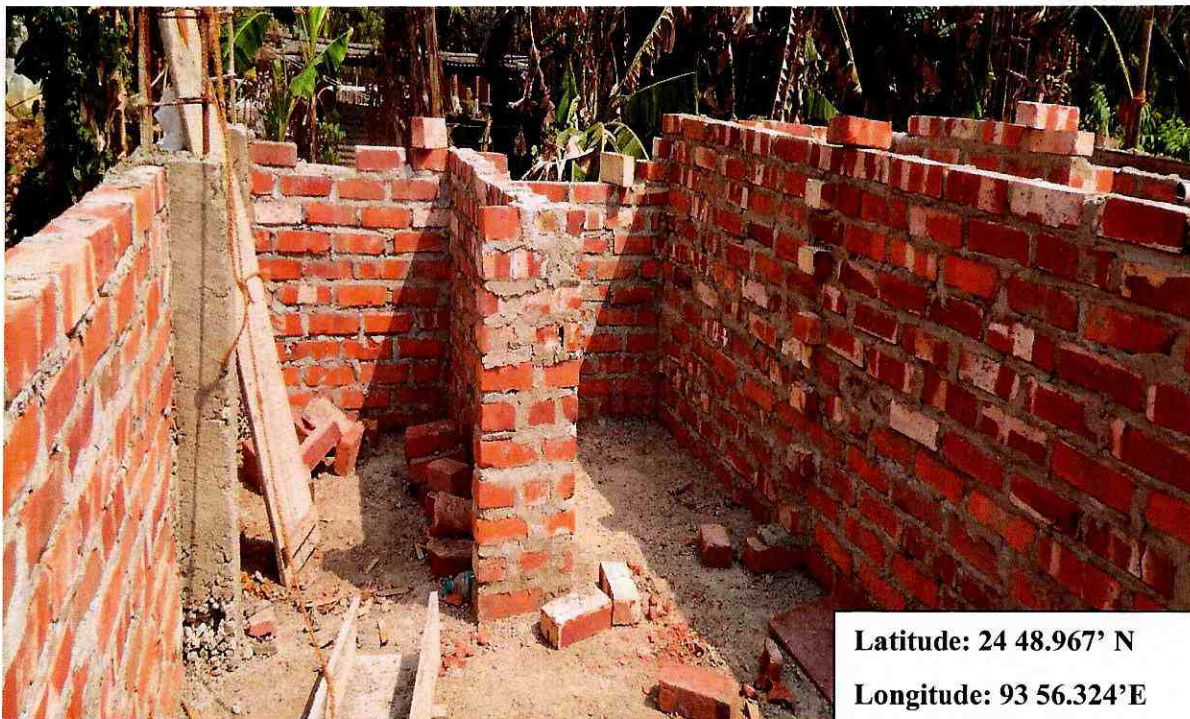
Photo of the details of the brickwork of the undergoing construction of the public toilets for the “Construction of Boys hostel (RCC+G2) with Toilets at Jawaharlal Nehru”, Manipur.
