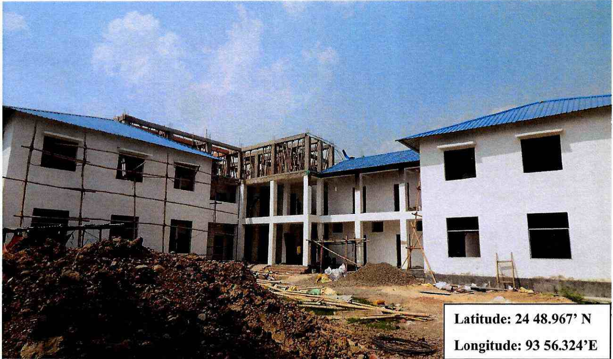
Overall view of the building for the "Construction of Boys hostel (RCC+G2) with Toilets at Jawaharlal Nehru", Manipur
