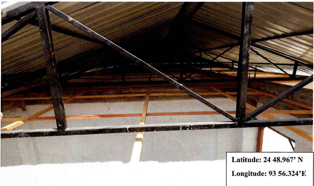
View showing the truss details of the roofing of the 1 st floor level of the building “Construction of Boys hostel (RCC+G2) with Toilets at Jawaharlal Nehru”, Manipur.
