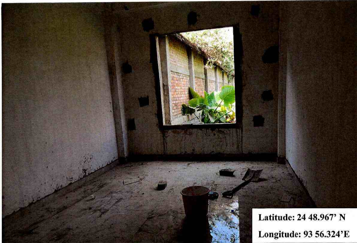
Photo showing the finishing work in progress of the rooms in the ground floor level of the building for the “Construction of Boys hostel (RCC+G2) with Toilets at Jawaharlal Nehru”, Manipur.
