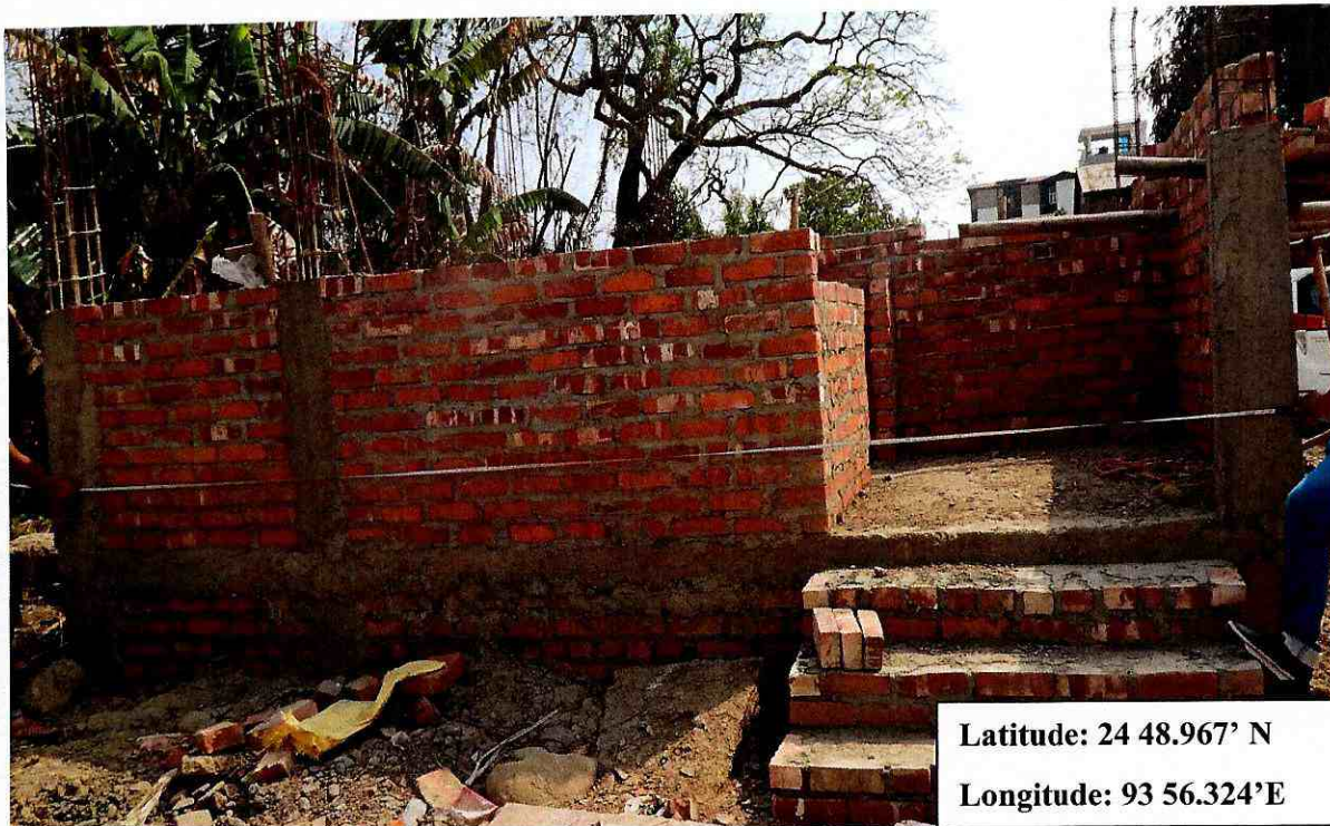
Photo of the undergoing construction of the public toilets for the “Construction of Boys hostel (RCC+G2) with Toilets at Jawaharlal Nehru”, Manipur.
