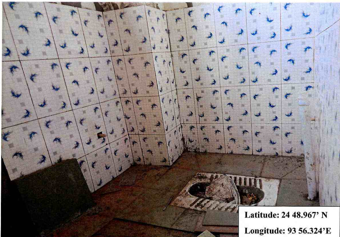
View inside the toilet showing the work in progress in the ground floor level inside the building for the “Construction of Boys hostel (RCC+G2) with Toilets at Jawaharlal Nehru”, Manipur.
