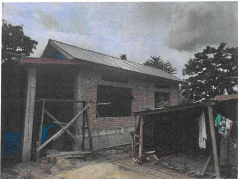
Overall view of "Construction of Transit Quarter for Doctors' and Nurses at Phoikon, Manipur."
