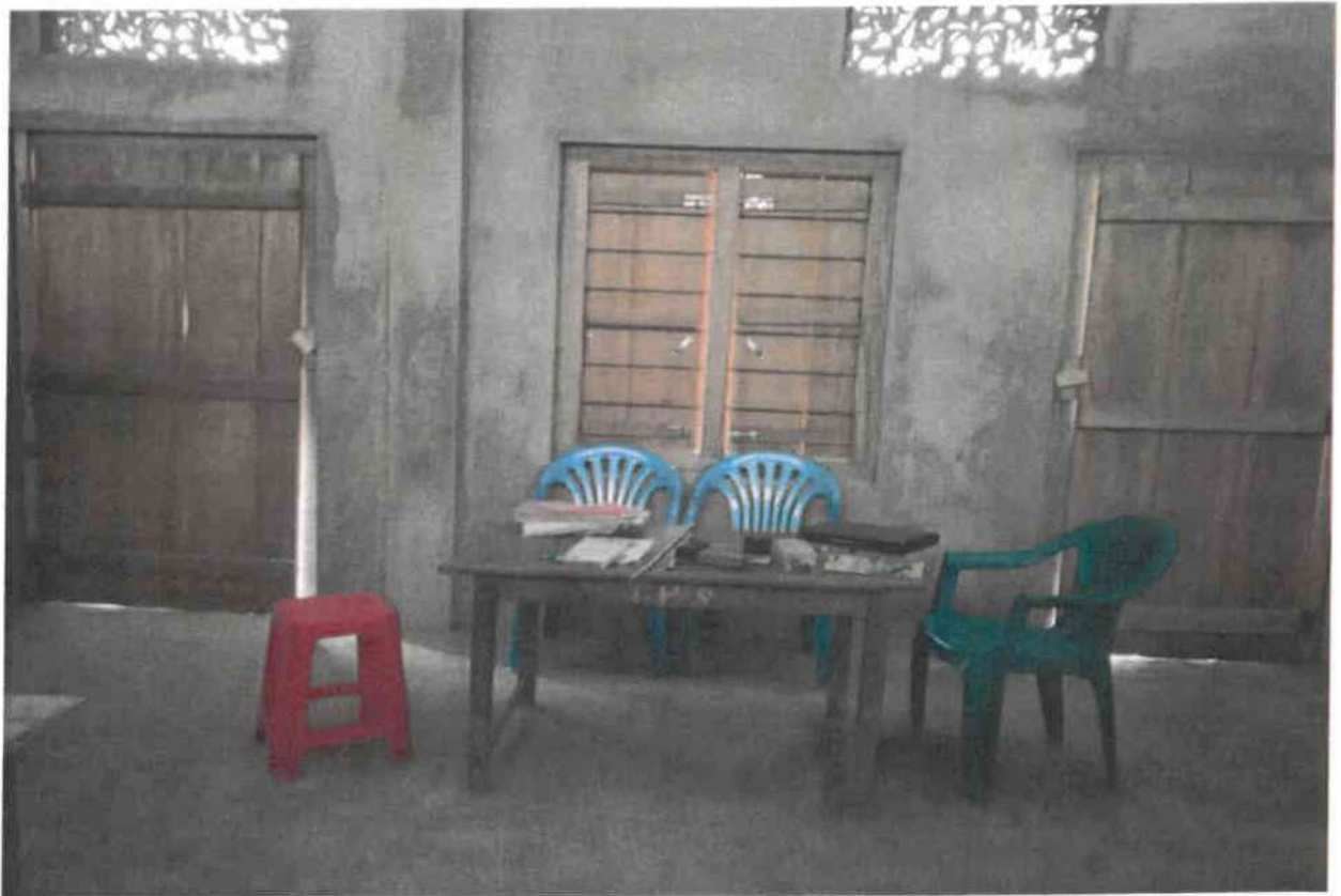
Inside view showing the doors and windows of "Construction of 2 additional Classrooms at Kovol Primary School, Tami, Manipur"
