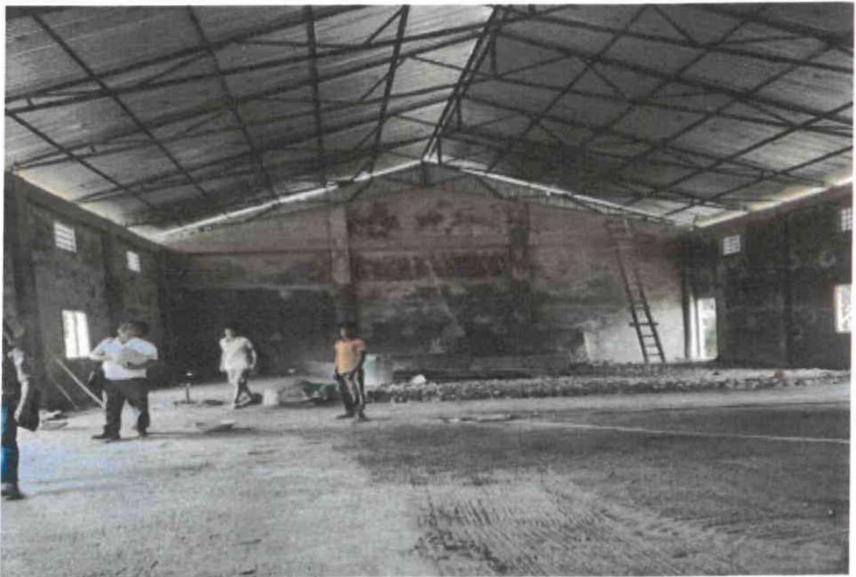
View inside the "Construction of Multipurpose Hall at Langching Sec. School, Manipur".
