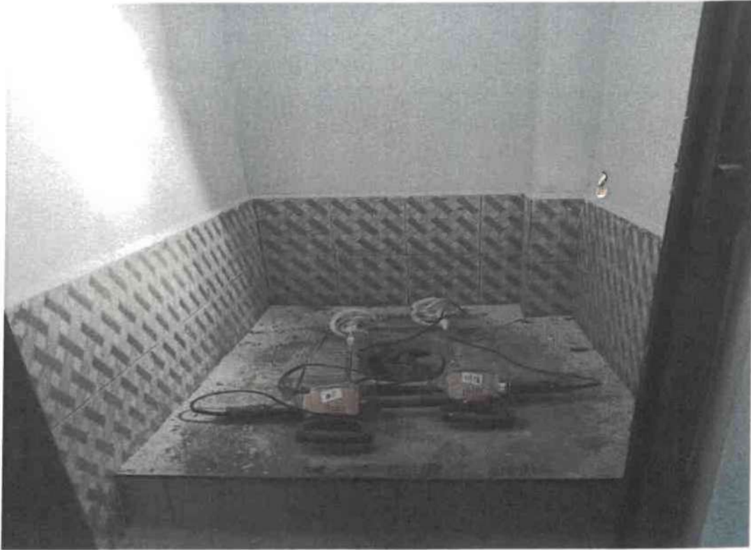
View inside the toilet of the “Construction of Teacher’s Transit Quarter at SDO Office Complex, Chakpikarong”
