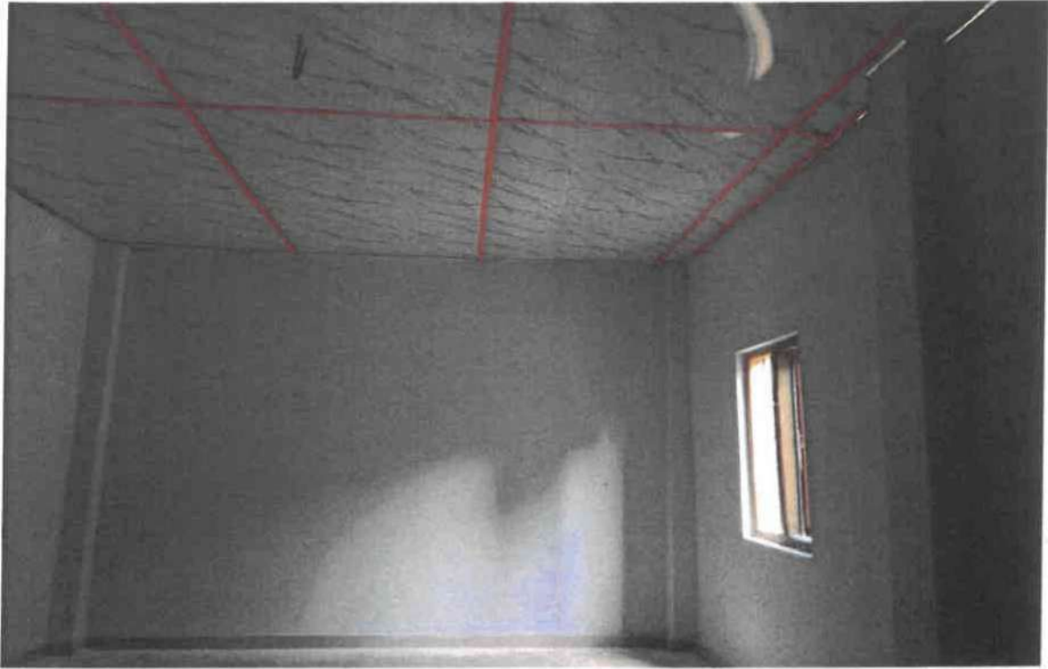
View inside the room for “Construction of Teacher’s Transit Quarter at SDO Office Complex, Chakpikarong”
