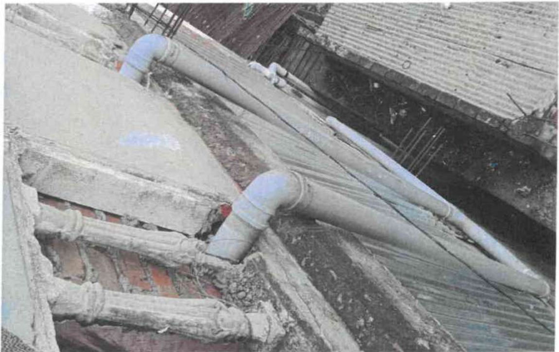
Photograph showing the sanitary pipelines for “Construction of Public Toilet at Chakikarong Bazar, Manipur”
