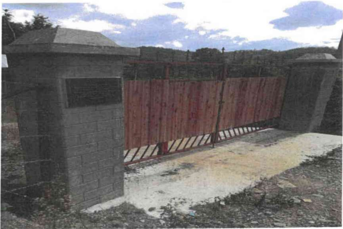
Photograph of the gate for "Construction of barb wire fencing with gate at Khubung Khunou Primary School, Manipur"
