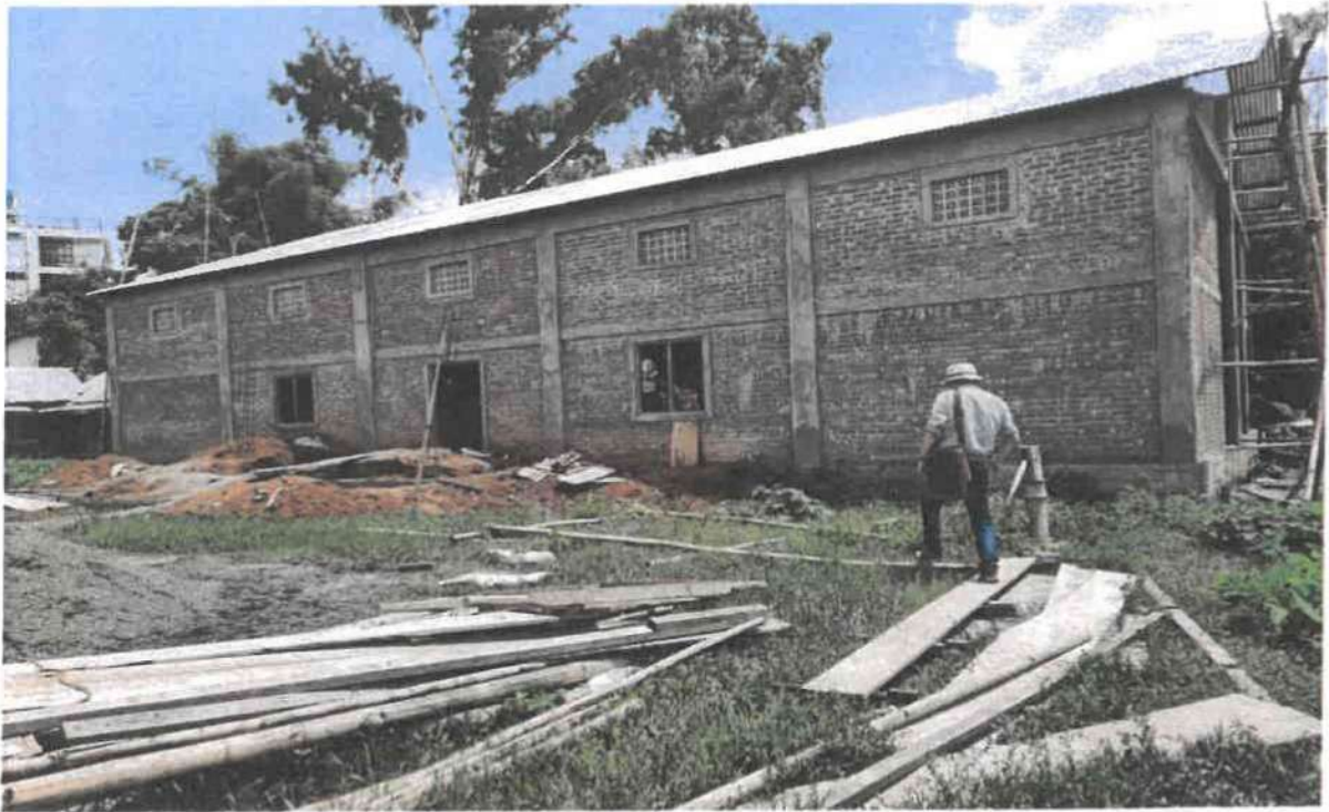
Overall view of the "Construction of Multipurpose Hall at Langching Sec. School, Manipur".
