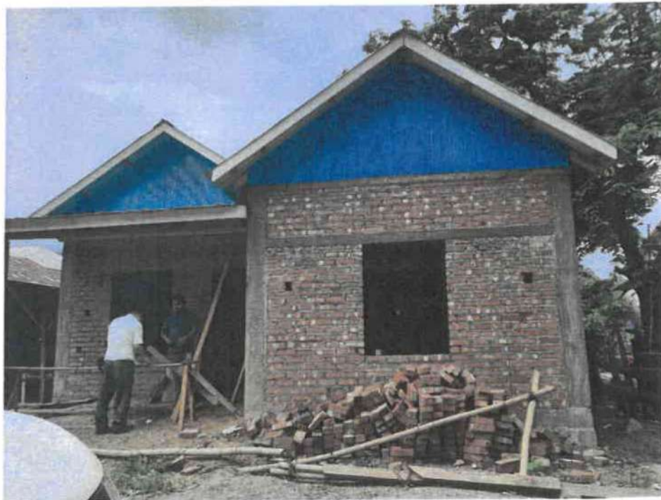
Overall view of "Construction of Teacher's Quarter at Sajik Tampak High School, Manipur"
