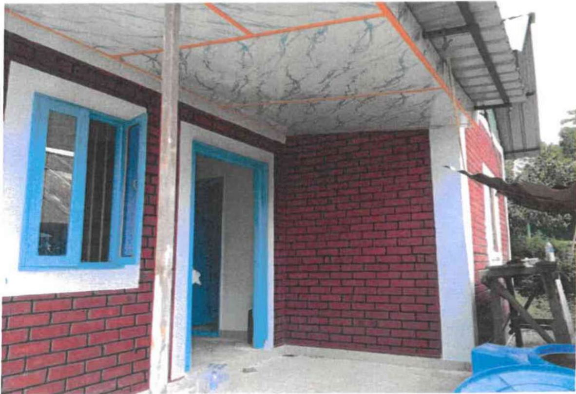
Front view of the "Construction of Teacher's Transit Quarter at SDO Office Complex, Chakpikarong"
