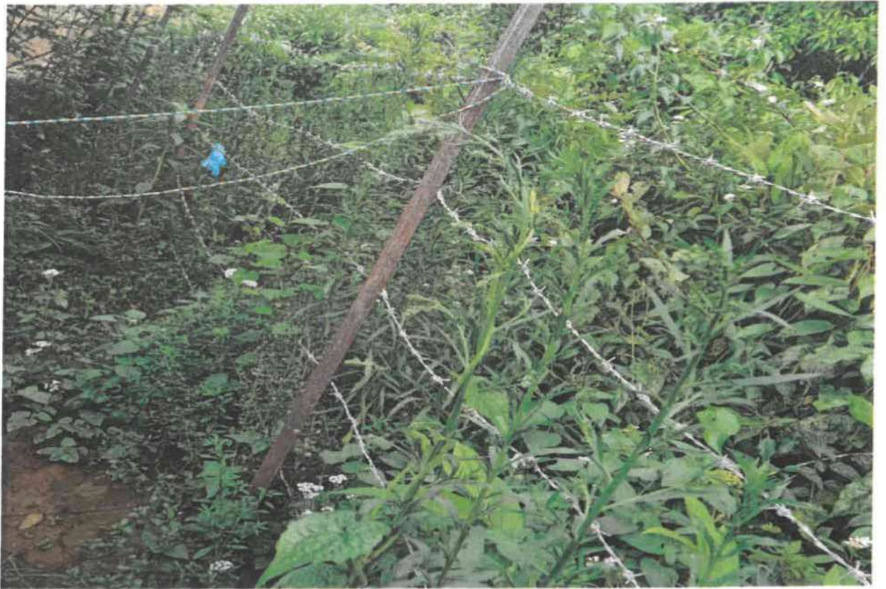
Photograph showing the barb wire fencing for the “Construction of barb wire fencing with gate at Khubung Khunou Primary School, Manipur”
