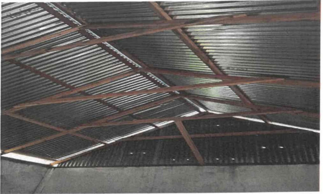
View showing the roofing/ceiling works of "Construction of 2 additional Classrooms at Kovol Primary School, Tami, Manipur"
