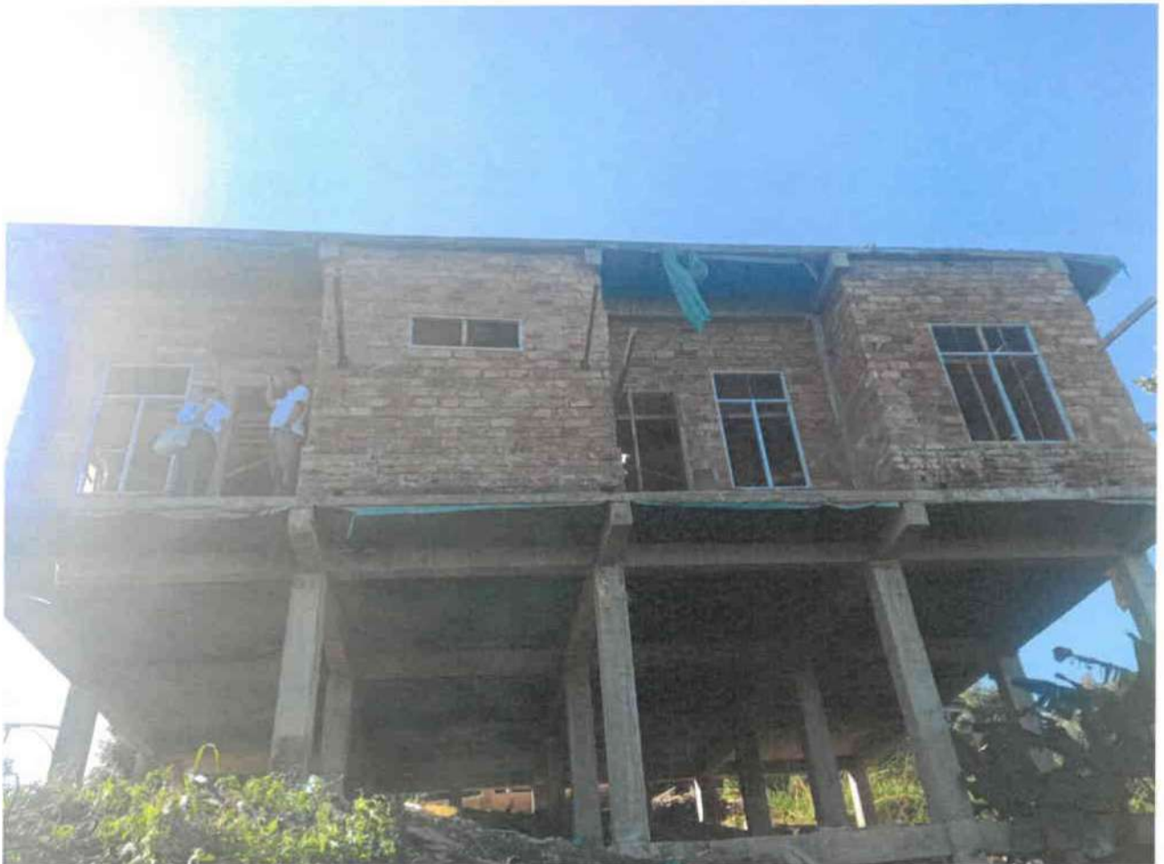
Back view of the building showing the basement of the building for the “Construction of Residential Quarters for BDO in Bungmun” .
