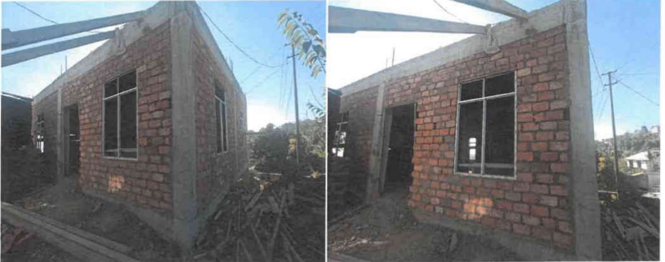
Overall view of the building for the “Construction of Residential Quarter for Medical Officer at Bunghmun” .
