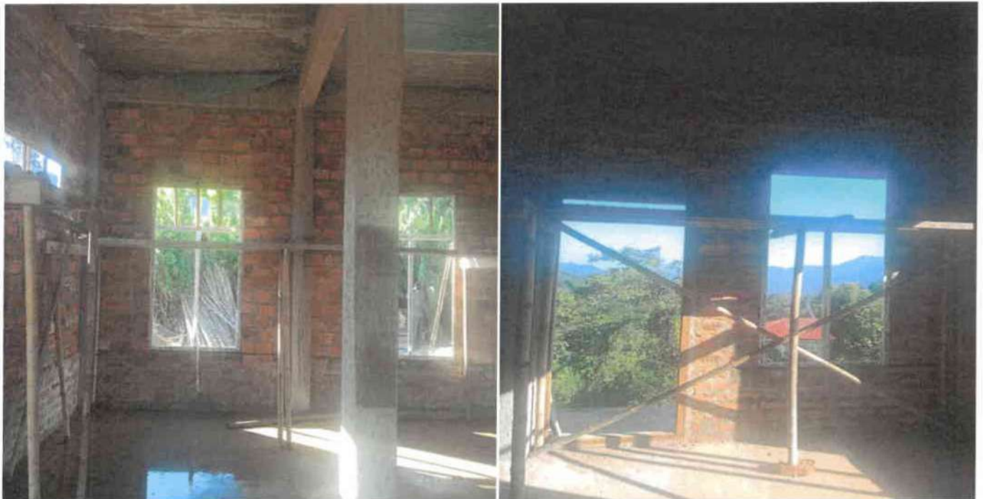
Photo showing the work in progress of the rooms of the building for the “ Construction of Residential Quarters for BDO in Bungmun ”.
