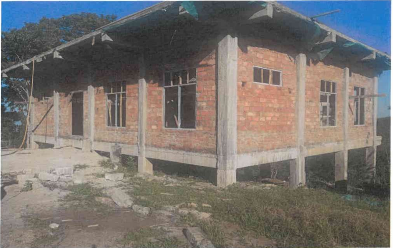
Overall view of the building for the “ Construction of Residential Quarters for BDO in Bungmun ”.
