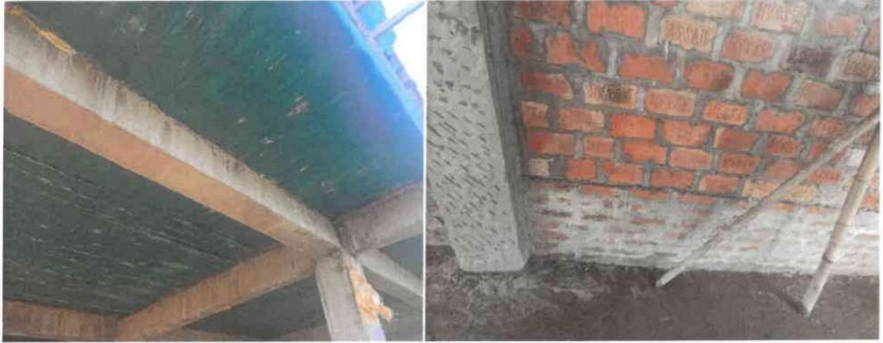
Photo showing the ceiling and the brickwork of the room of the building for the “Construction of Residential Quarters for BDO in Bungmun” .
