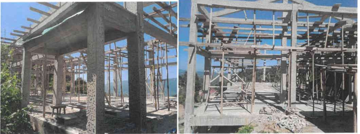
Photo showing the work in progress of the building for the “Construction of Community Hall at Buarpui” .
