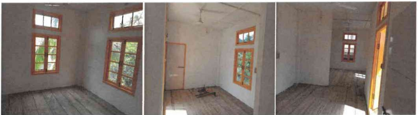
View inside the rooms of the building for the “Construction of Sub-Centre Building at Thenlum.”
