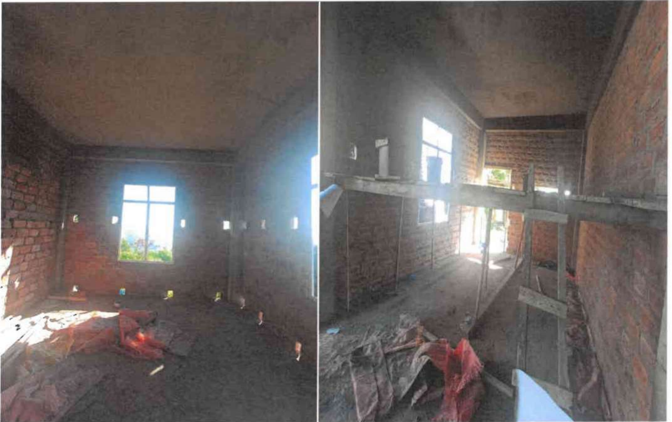
Photo showing the work in progress of the rooms of the building for the “Construction of Residential Quarter for Medical Officer at Bunghmun” .
