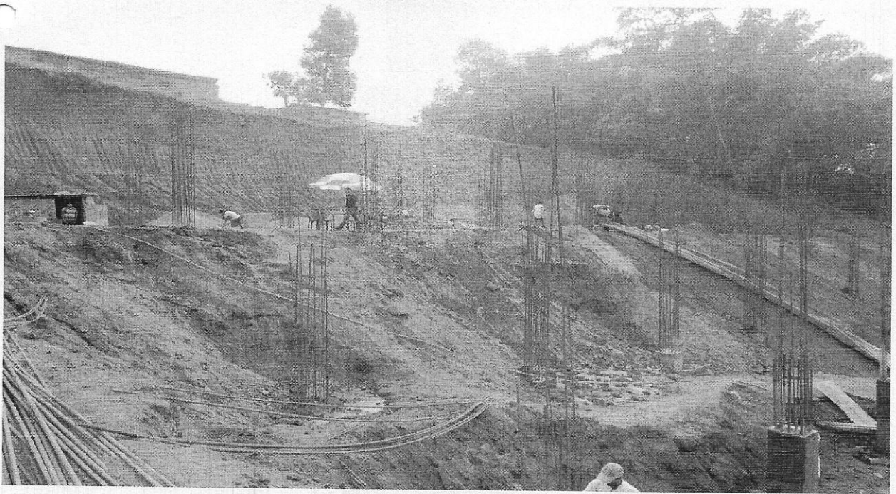
View of ongoing construction work for the Institute Building at Omeo Kumar Das Institute of Social Change and Development, Guwahati
