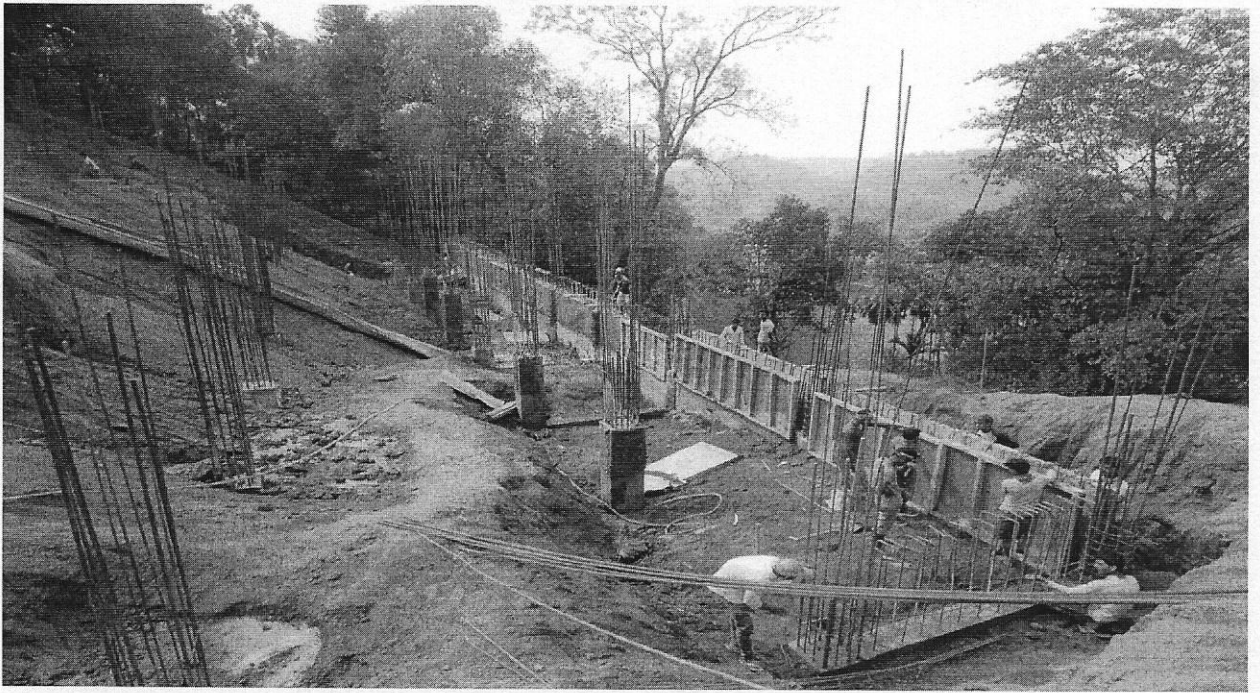
View of the ongoing construction work at Omeo Kumar Das Institute of Social Change and Development , Guwahati
