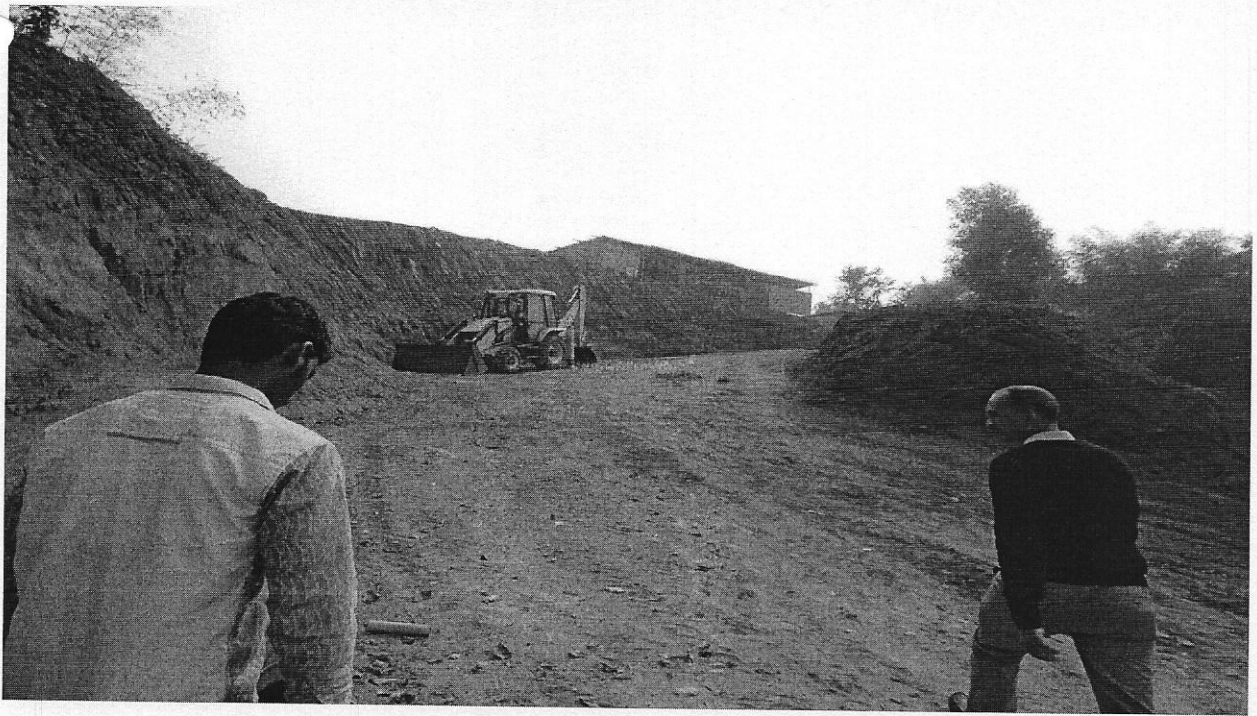
View of construction of Internal Road at Omeo Kumar Das Institute of Social Change and Development, Guwahati
