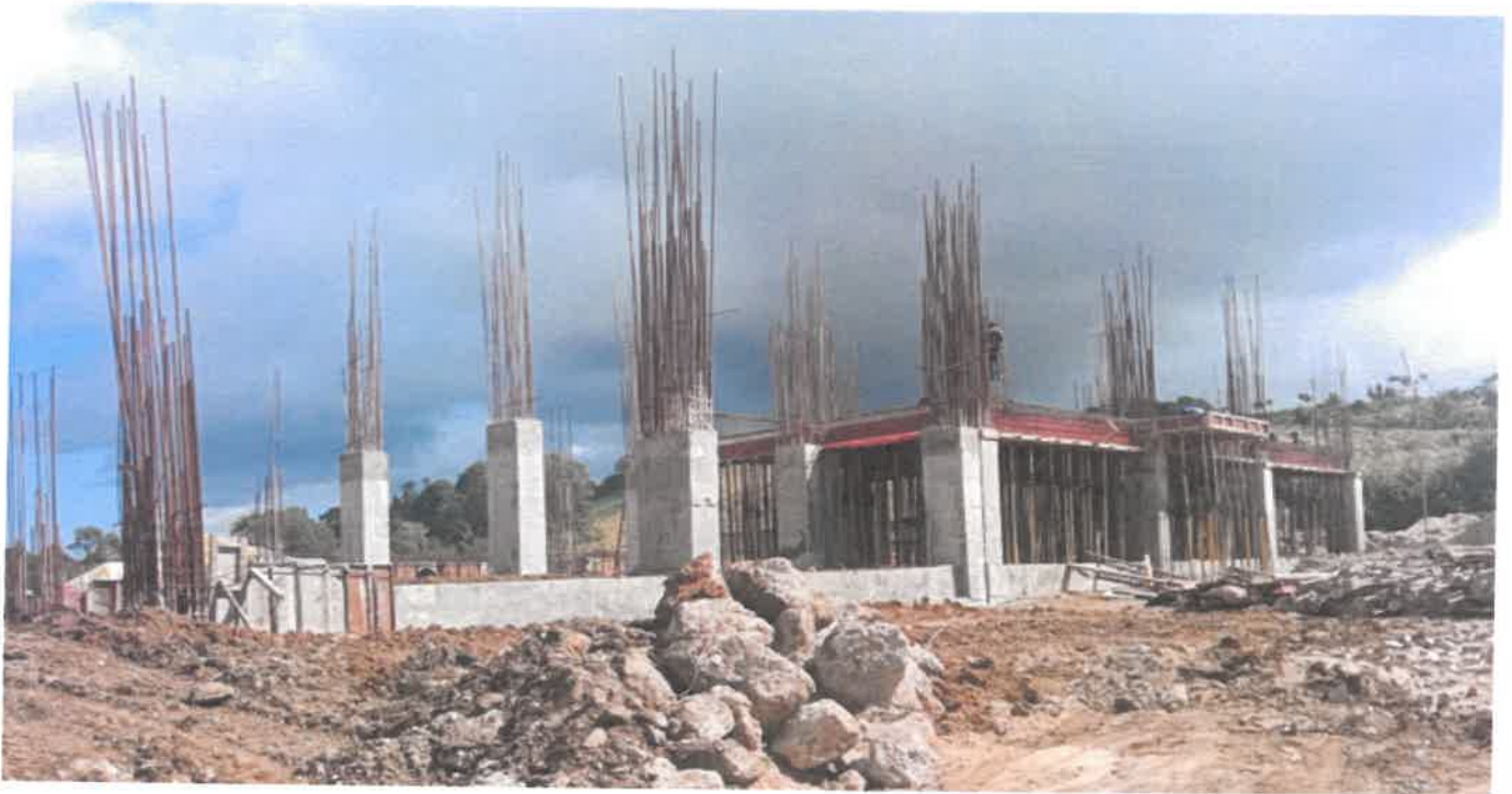
Side view of the work in progress for the indoor stadium of the "Construction of Indoor Stadium at Madan Tukhon, Jongsha Meghalaya."
