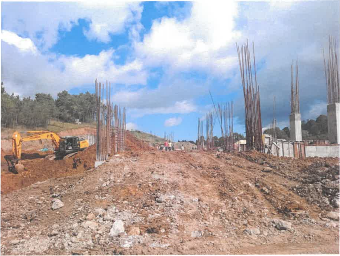
Photograph showing the excavation work in progress of the indoor stadium of the “Construction of Indoor Stadium at Madan Tukhon, Jongsha Meghalaya”.
