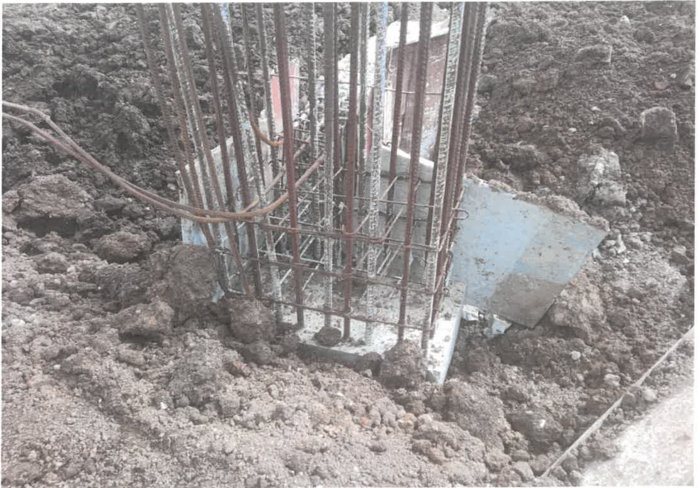
Photograph showing reinforcement detailing of the indoor stadium of the "Construction of Indoor Stadium at Madan Tukhon, Jongscha Meghalaya".
