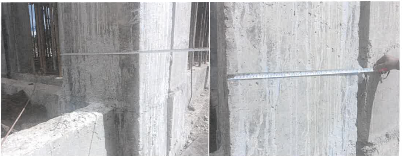
Photograph showing the inspection team taking the measurement of components of the indoor stadium of the “Construction of Indoor Stadium at Madan Tukhon, Jongsha Meghalaya”.
