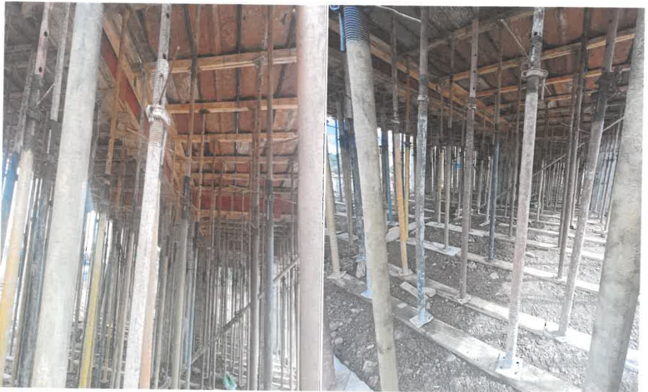
Photograph showing the form work in progress for Part I of the indoor stadium of the "Construction of Indoor Stadium at Madan Tukhon, Jongsha Meghalaya."
