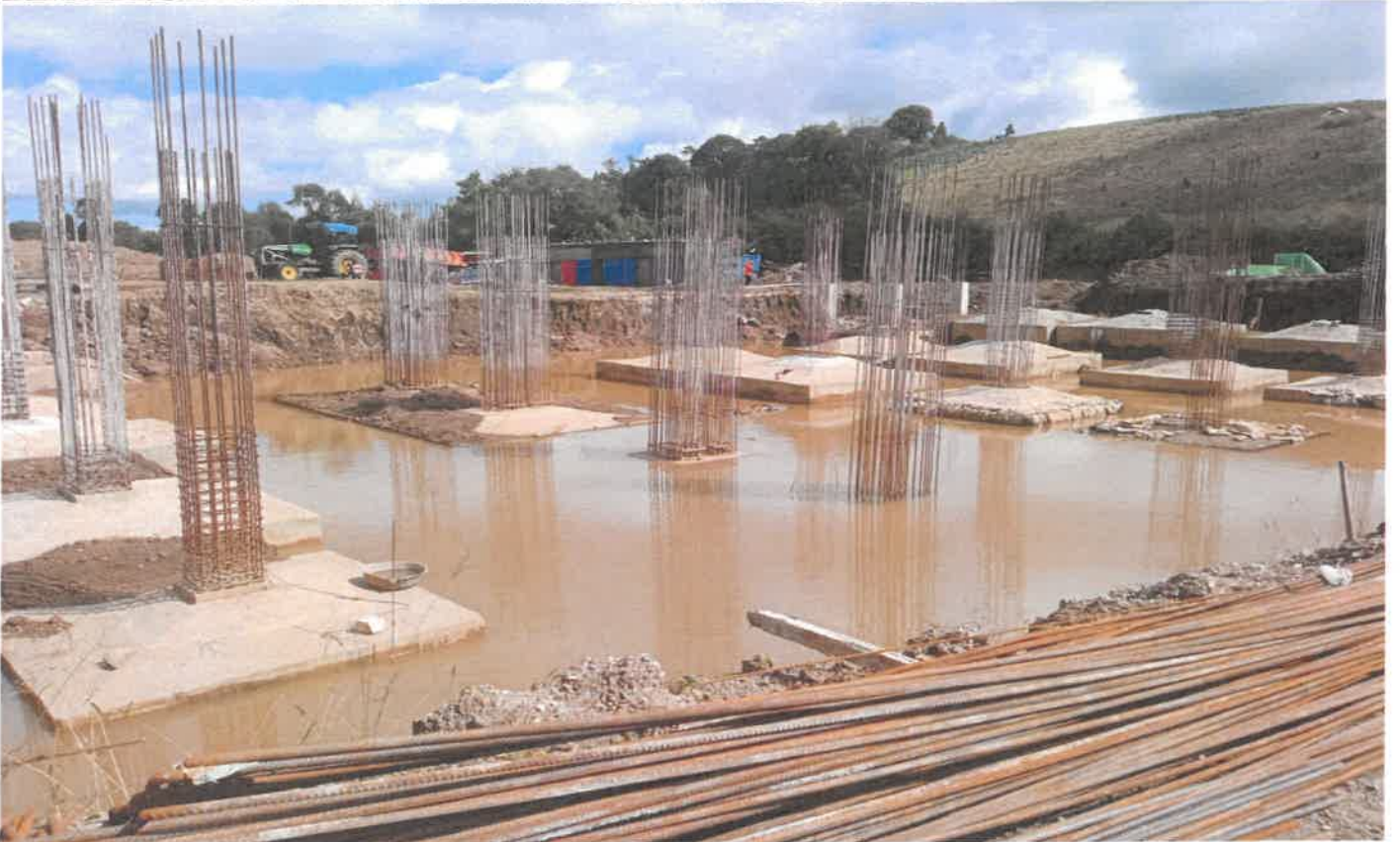
Photograph showing foundation work in progress for the other portion of the indoor stadium of the "Construction of Indoor Stadium at Madan Tukhon, Jongshe Meghalaya".
