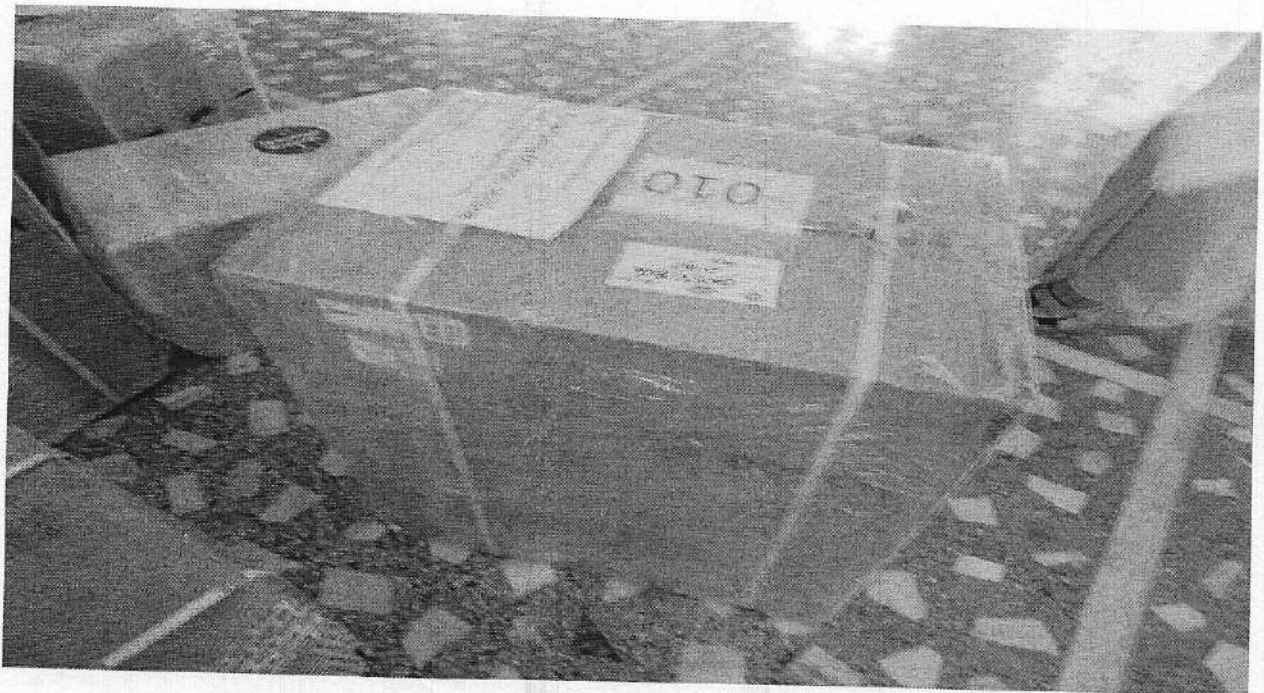
View of Servers stored in the Store room
