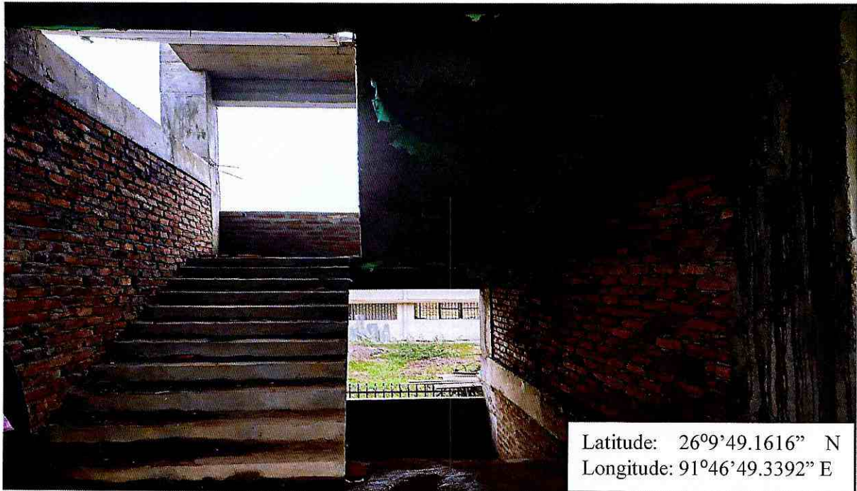
View of the staircase towards the 1 st floor level for the “Construction of Composite Regional Centre(North East) for Disability Study and Action in Assam by Shishu Sarothi”
