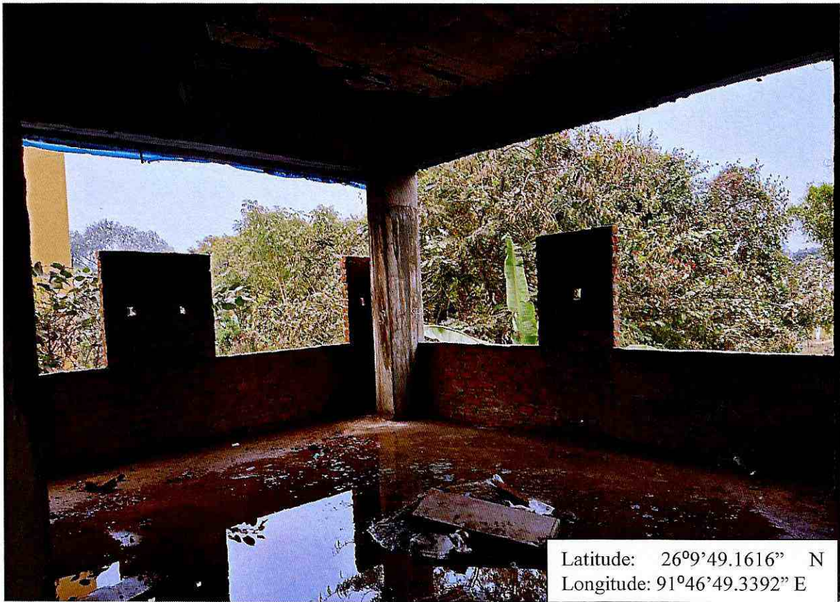
Brickwork in progress in the 1 st floor level for the “Construction of Composite Regional Centre(North East) for Disability Study and Action in Assam by Shishu Sarothi”
