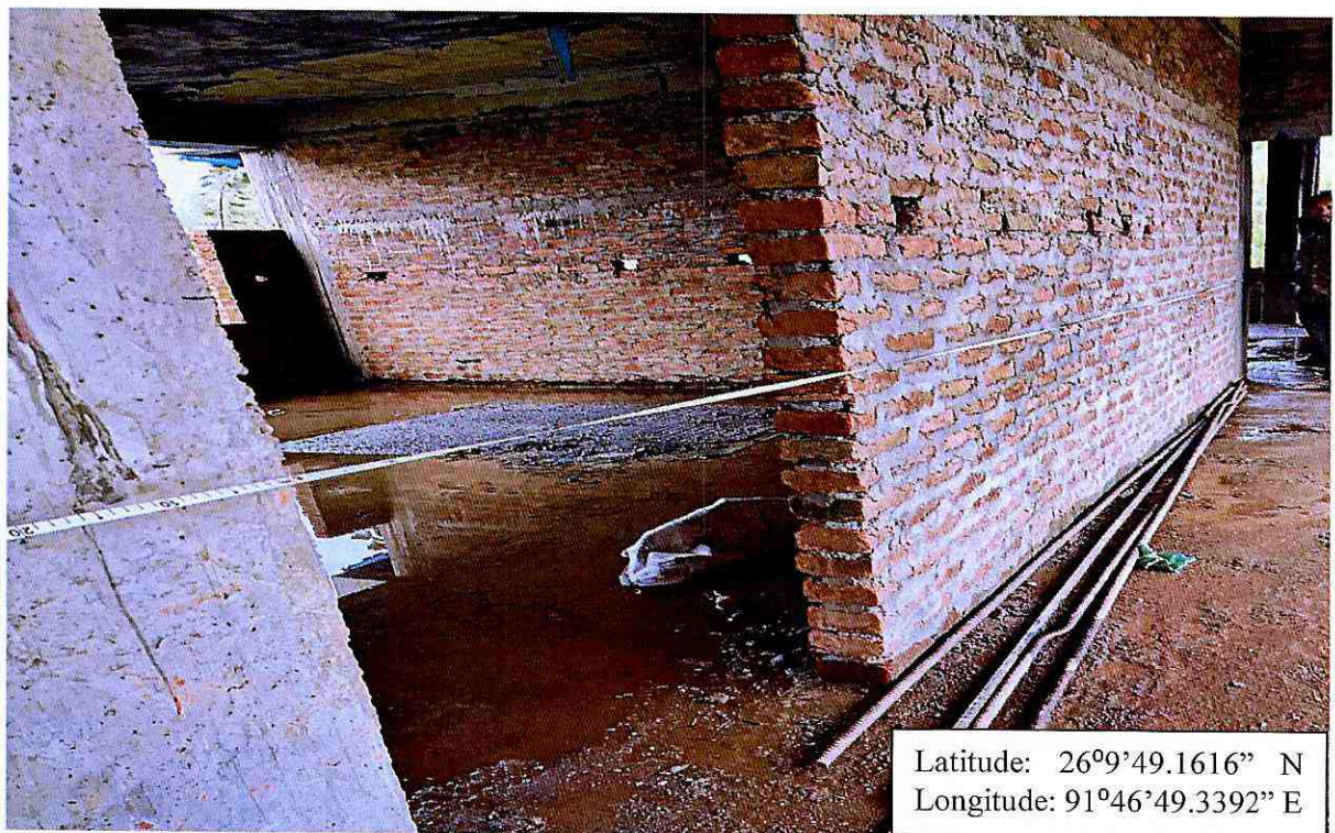
Photo of the ongoing work of classroom for the “Construction of Composite Regional Centre(North East) for Disability Study and Action in Assam by Shishu Sarothi”
