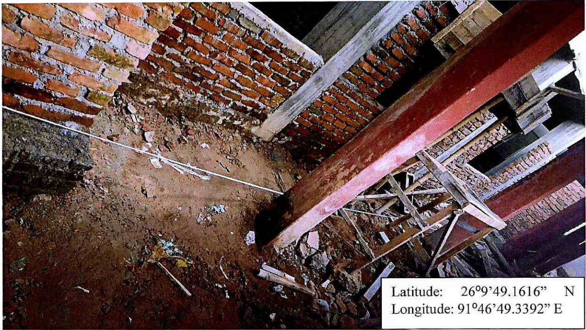
Brickwork in the Ground floor level for the “Construction of Composite Regional Centre(North East) for Disability Study and Action in Assam by Shishu Sarothi”
