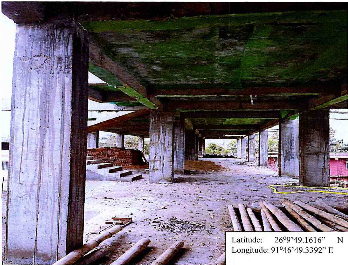
View inside the 2 nd floor level for the "Construction of Composite Regional Centre(North East) for Disability Study and Action in Assam by Shishu Sarothi"
