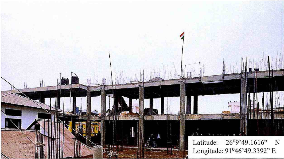
View of the building for the "Construction of Composite Regional Centre(North East) for Disability Study and Action in Assam by Shishu Sarothi"
