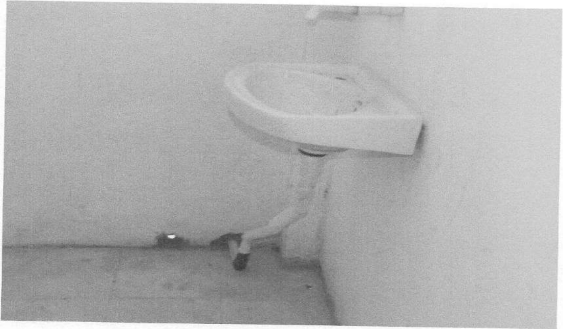
A view of the sink without proper tap .
