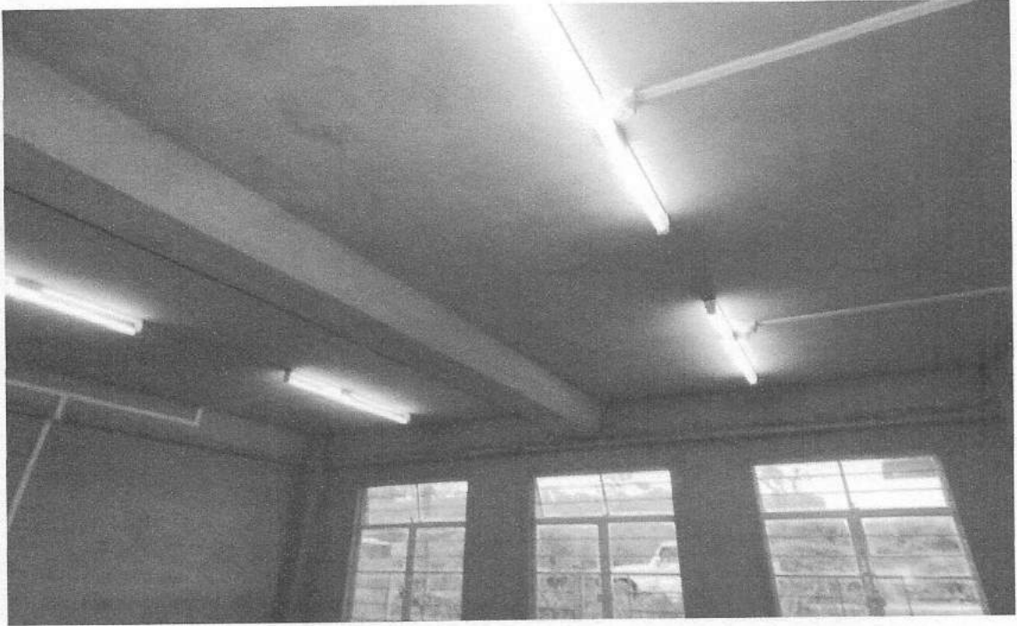
A view of the interior of a room along with the electrical work.
