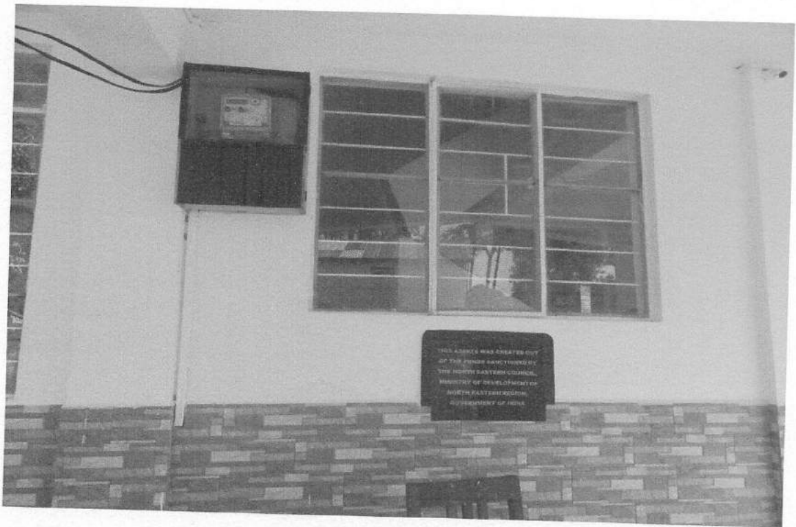
A view of the meter box with the plaque stating that NEC has funded the project
