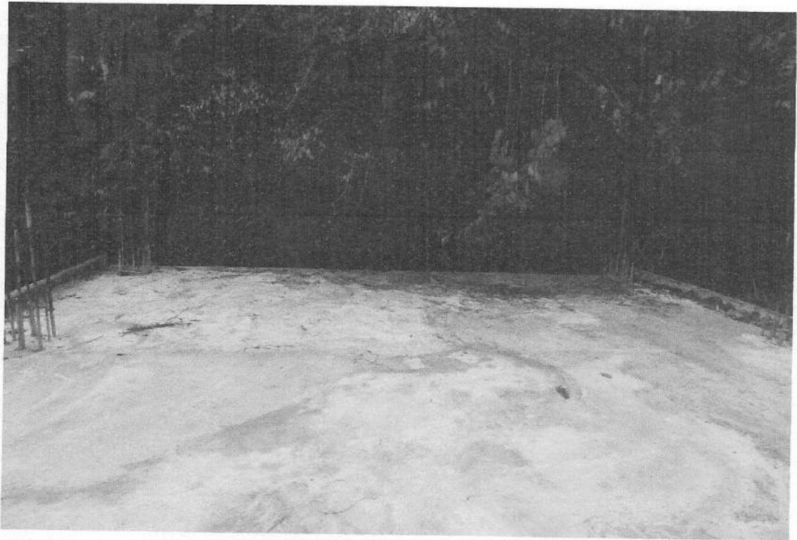
No roof protection found.
