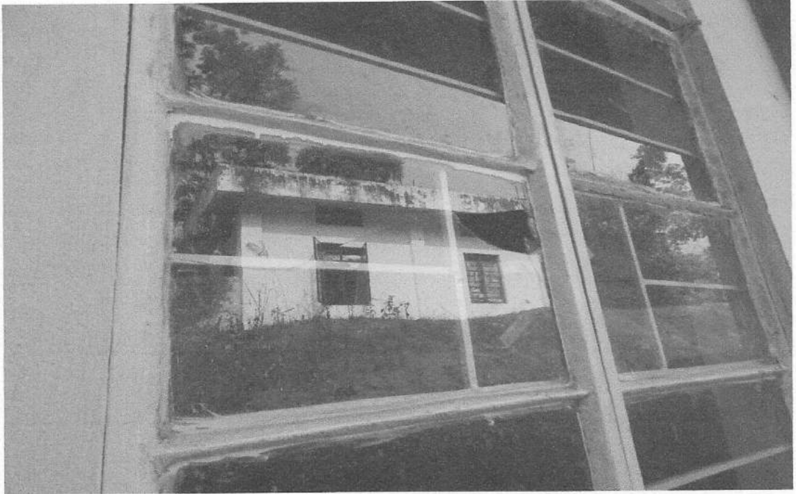
A view of the broken glass on the window.
