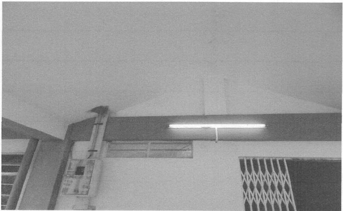
The porch and the Meter Box at the entrance.
