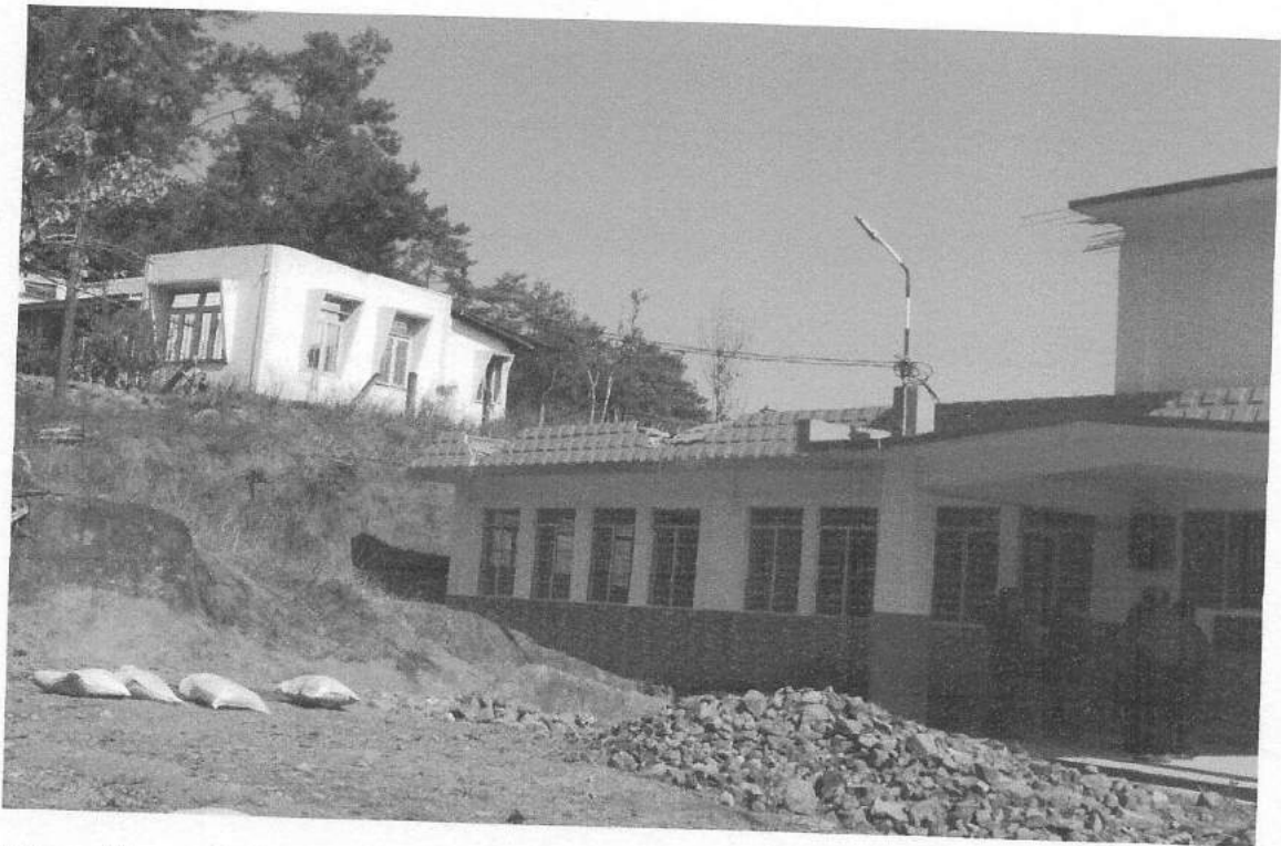
A view of the cracked wall on the terrace .
