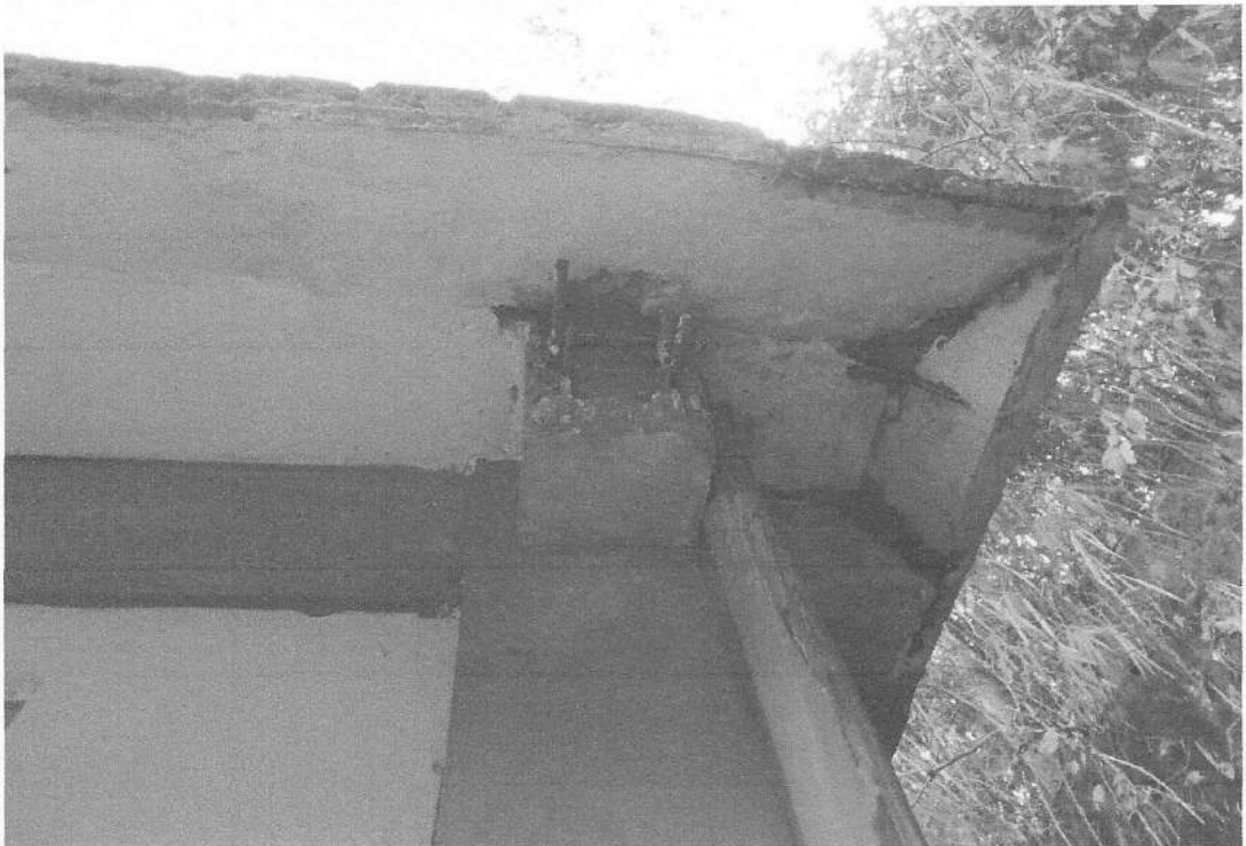
A view of cracks found on the exterior wall.
