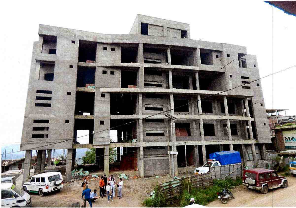
1. Photo of the building of the Setting up of Multi- Disciplinary Livelihood Incubation centre for Food Processing, Ready Garment making and Handicraft at Hunpun, Ukhrul
