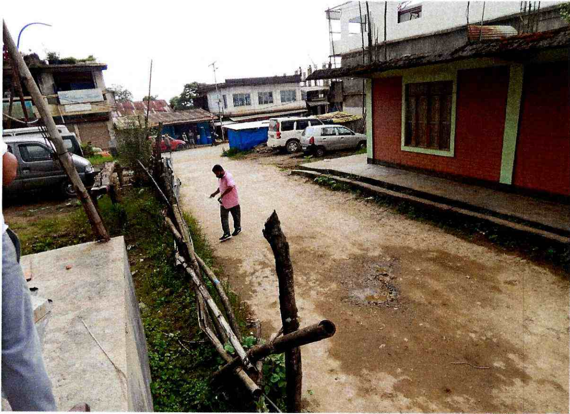
7. View of the approach Road and pathway of Multi-Disciplinary Livelihood Incubation centre for Food Processing, Ready Garment making and Handicraft at Hunpun, Ukhrul
