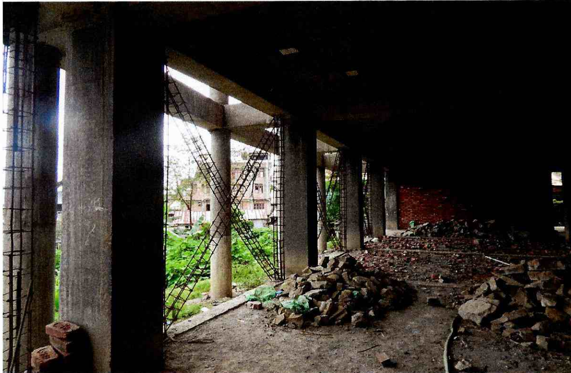
3. Photo of work in progress of ground floor of Multi- Disciplinary Livelihood Incubation centre for Food Processing, Ready Garment making and Handicraft at Hunpun, Ukhrul
