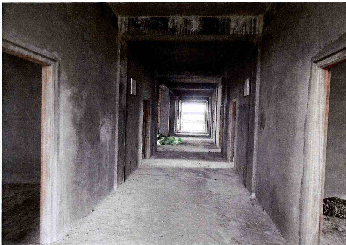
5. View of the Corridor of the 3 rd floor of Multi- Disciplinary Livelihood Incubation centre for Food Processing, Ready Garment making and Handicraft at Hunpun, Ukhrul
