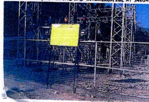
SWITCH YARD WITH SIGN BOARD AT YANGANG.
